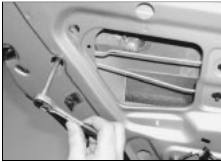
13.13a Unscrew the nuts, using a socket inserted through the aperture provided . . .
