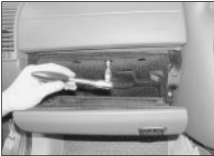
31.3 Slacken and withdraw the screws that secure the lower edge of the passenger airbag unit cover panel to the fascia
