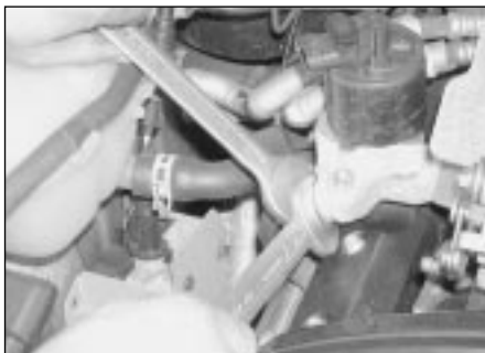
15.35a Unscrew the union nut and free the EGR pipe from the EGR valve
