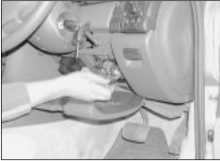
3.2 The main fuses and relays are located in a panel beneath a cover under the driver's side of the facia
