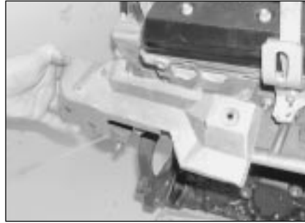
6.45b . . . and upper heatshields from the right-hand exhaust manifold (shown with engine removed)
