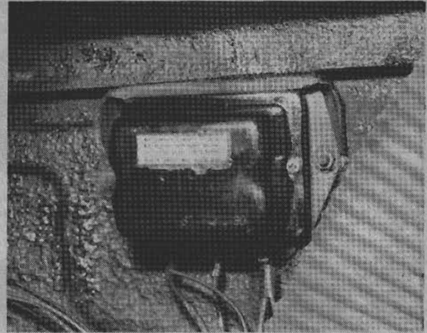
Fig. 8.7. The control box showing the terminal numbering
