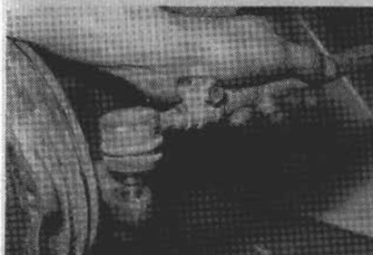
6.6. Undo the ball joint from steering arm. It may need a judicious blow with a hammer to jolt it out
