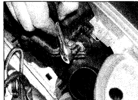
2.9a To remove the air cleaner, undo the bolt at the front . . .
