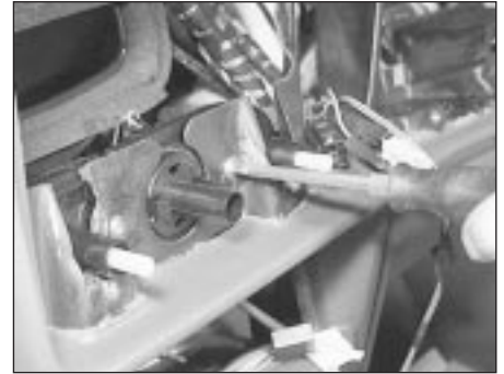
41.19 Undo the heater control panel retaining screws and free the panel from the fascia
