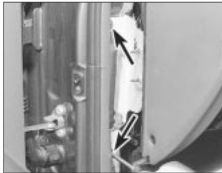
41.35a Partially withdraw the facia to gain access to left-hand support bracket retaining screws (arrowed) . . .
