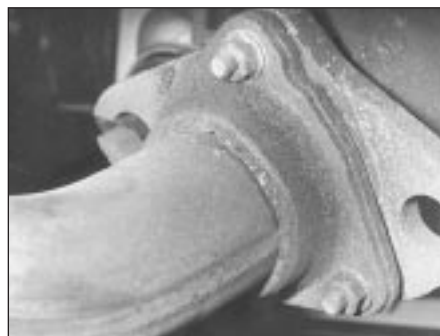
18.6 Front pipe-to-manifold flange joint
