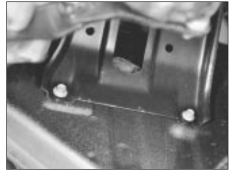
4.6b Battery tray mounting bracket retaining bolts (viewed from underneath)
